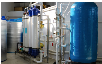
Water filtration systems
